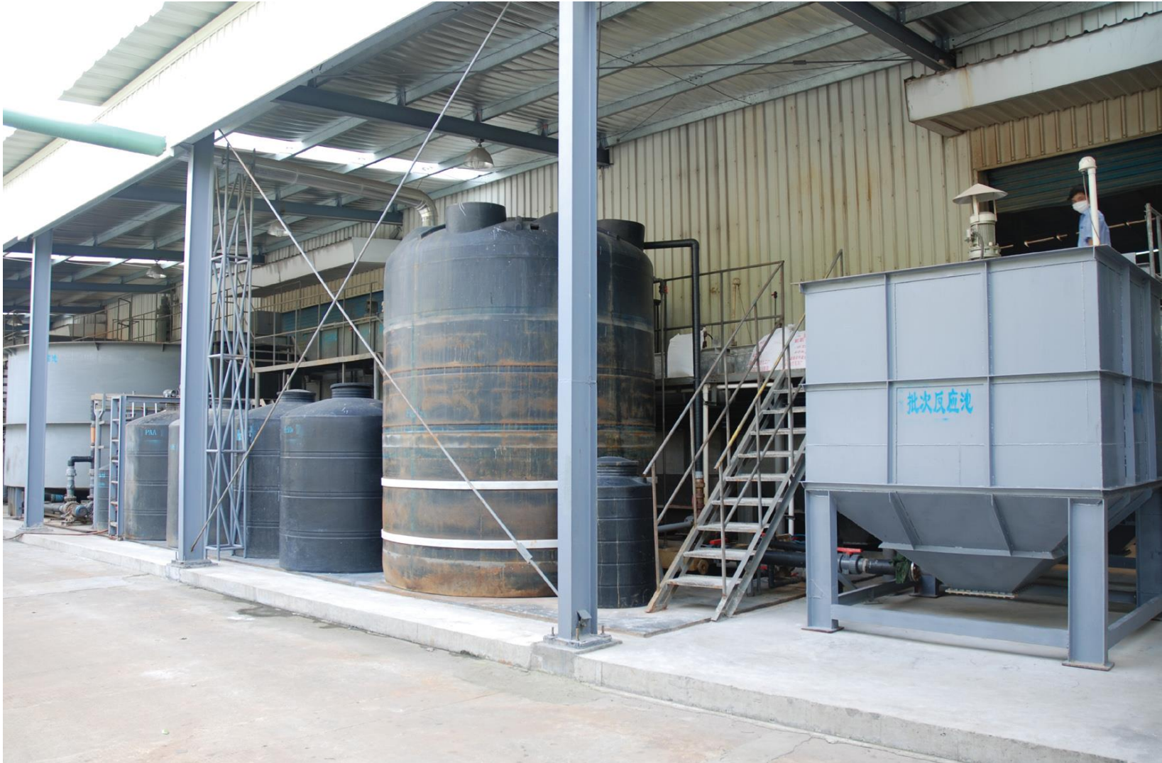
New exhaust gas treatment
