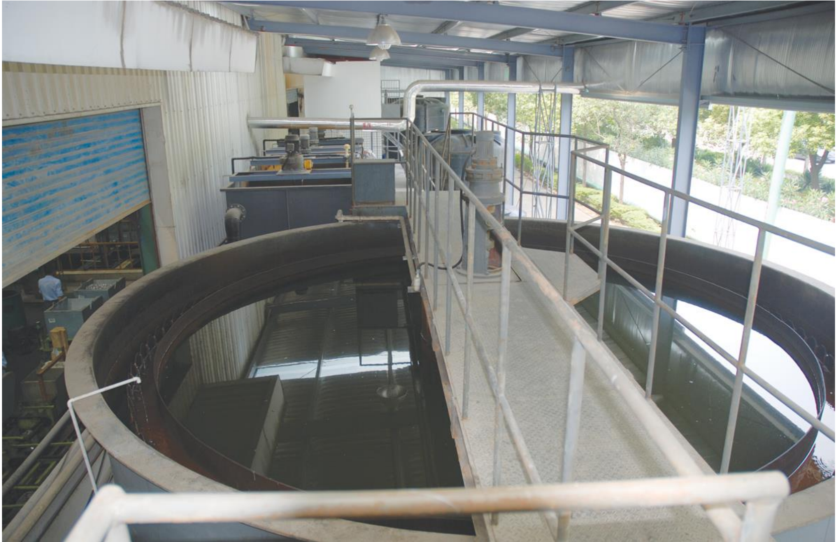
New exhaust gas treatment
