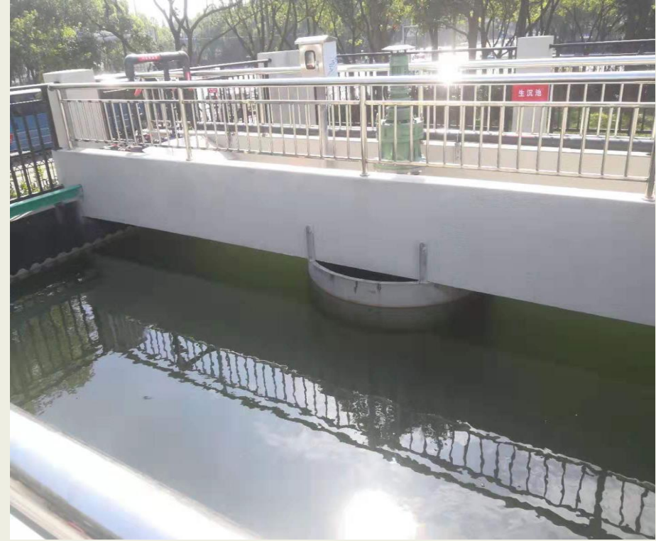
New sewage processing station
